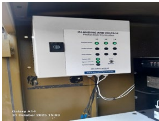
Figure 2: Controller installed in MV switchgear enclosure
