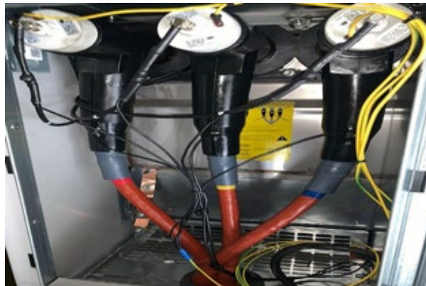
Figure 2: 24 kV OAS sensor installed in cable compartment (T-plug connection)
