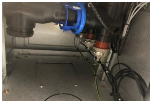
Figure 3: 12 kV OAS sensor mounted on busbar chamber (elbow connector)
